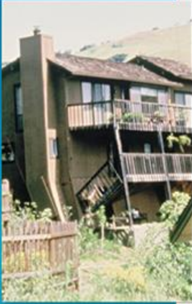
The balcony of this hillside home partially collapsed and the home tilted when the stilt-type support posts and poorly braced walls shifted during an earthquake.
