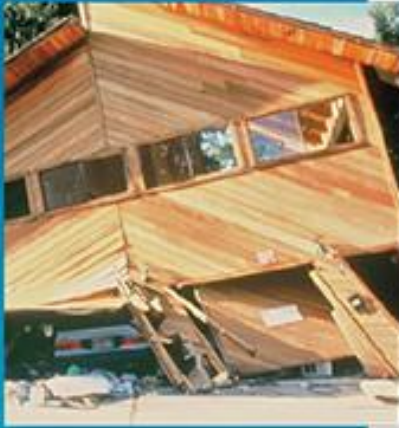
The walls around the garage door of this home were not strong enough to withstand the shaking of the 1989 Loma Prieta Earthquake.
